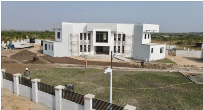
Exterior View (Front): Plastering and painting on the building has been completed.
